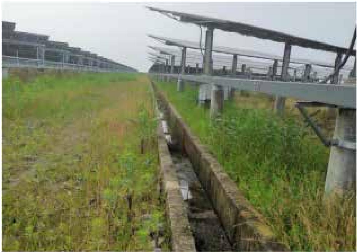
Figure 11 Drainage ditch under photovoltaic panels
