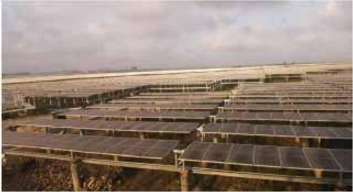
Figure 3 Photovoltaic power generation area
