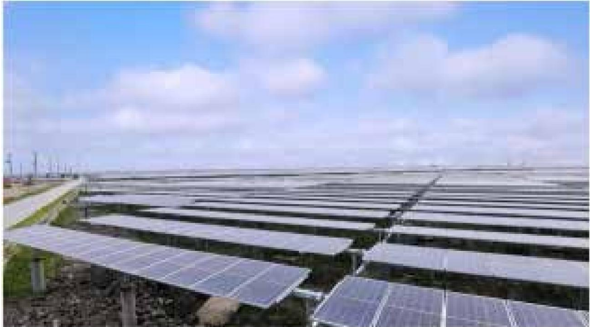
Figure 1 Photovoltaic power generation area
