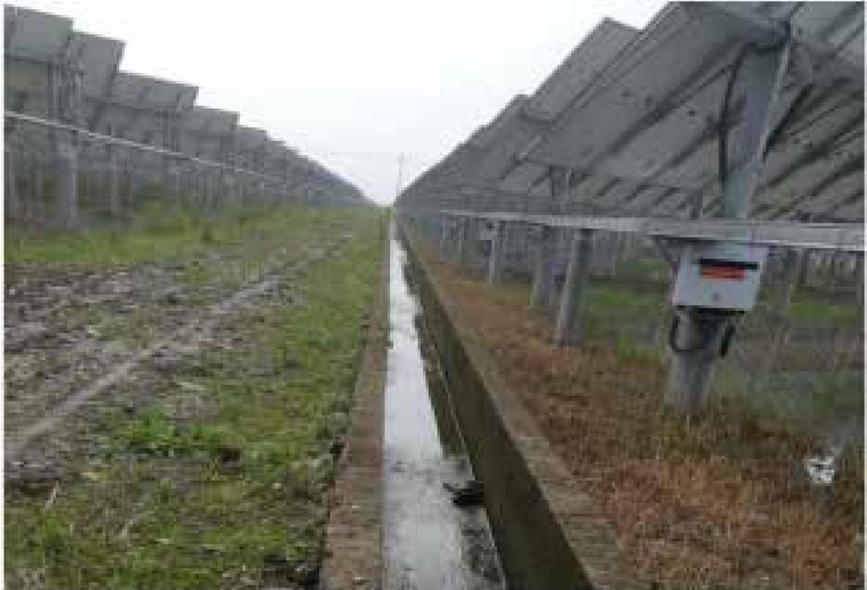
Figure 10 Drainage ditch under photovoltaic panels
