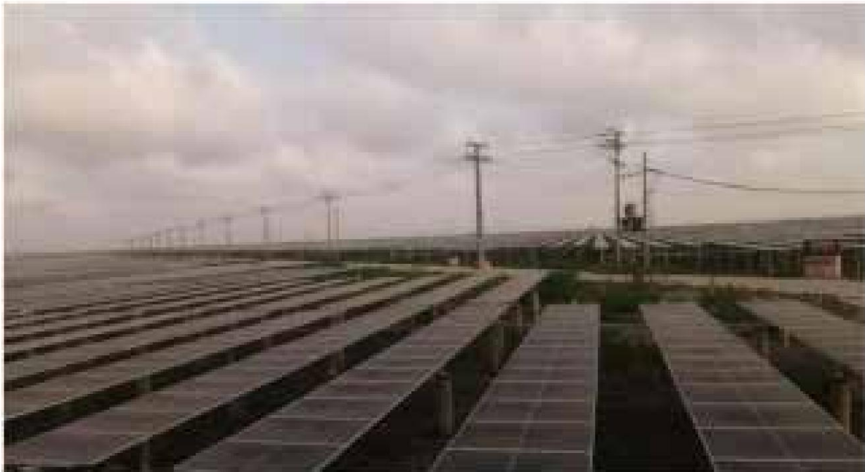
Figure 2 Photovoltaic power generation area
