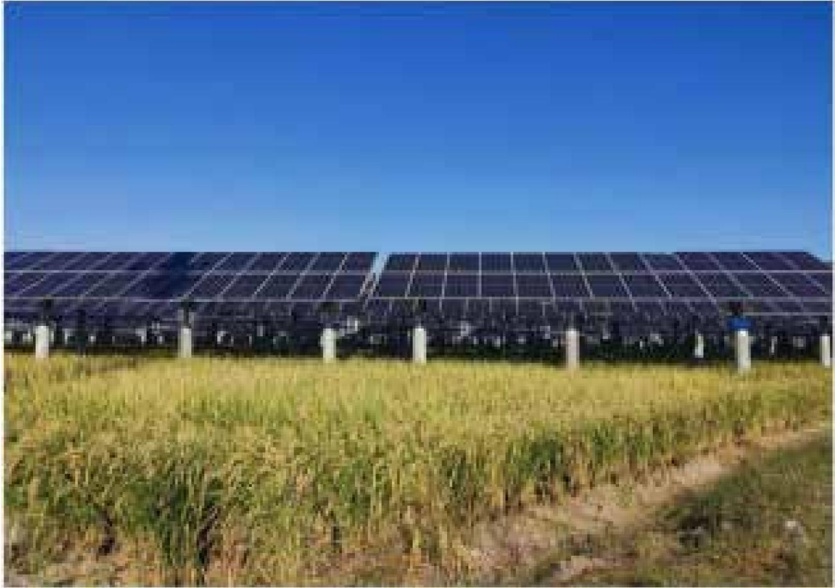
Figure 9: Recultivation under photovoltaic panels
